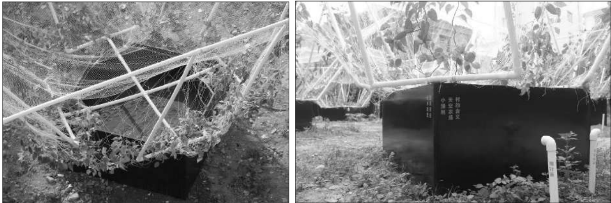
Figure 6. Rainwater Storage Tank Of Sky Farm Installation (URL 6).
